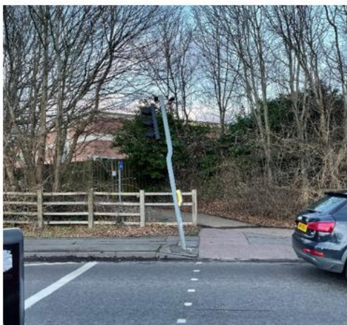
Leaning traffic signal pole before refurbishment
