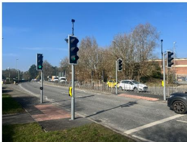
Refurbished Traffic signal at Portfield Way, Chichester
